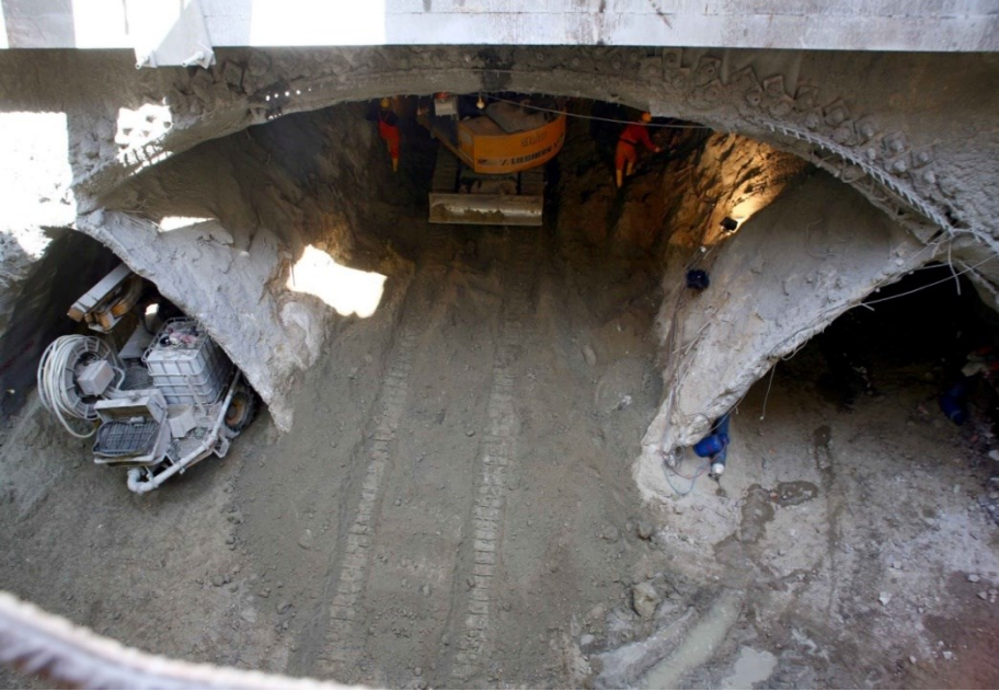
Construction of a station using an arch structure according to the New Austrian Tunneling Method /MS Serdika II/
